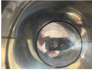
Damper Flap in Closed Position
